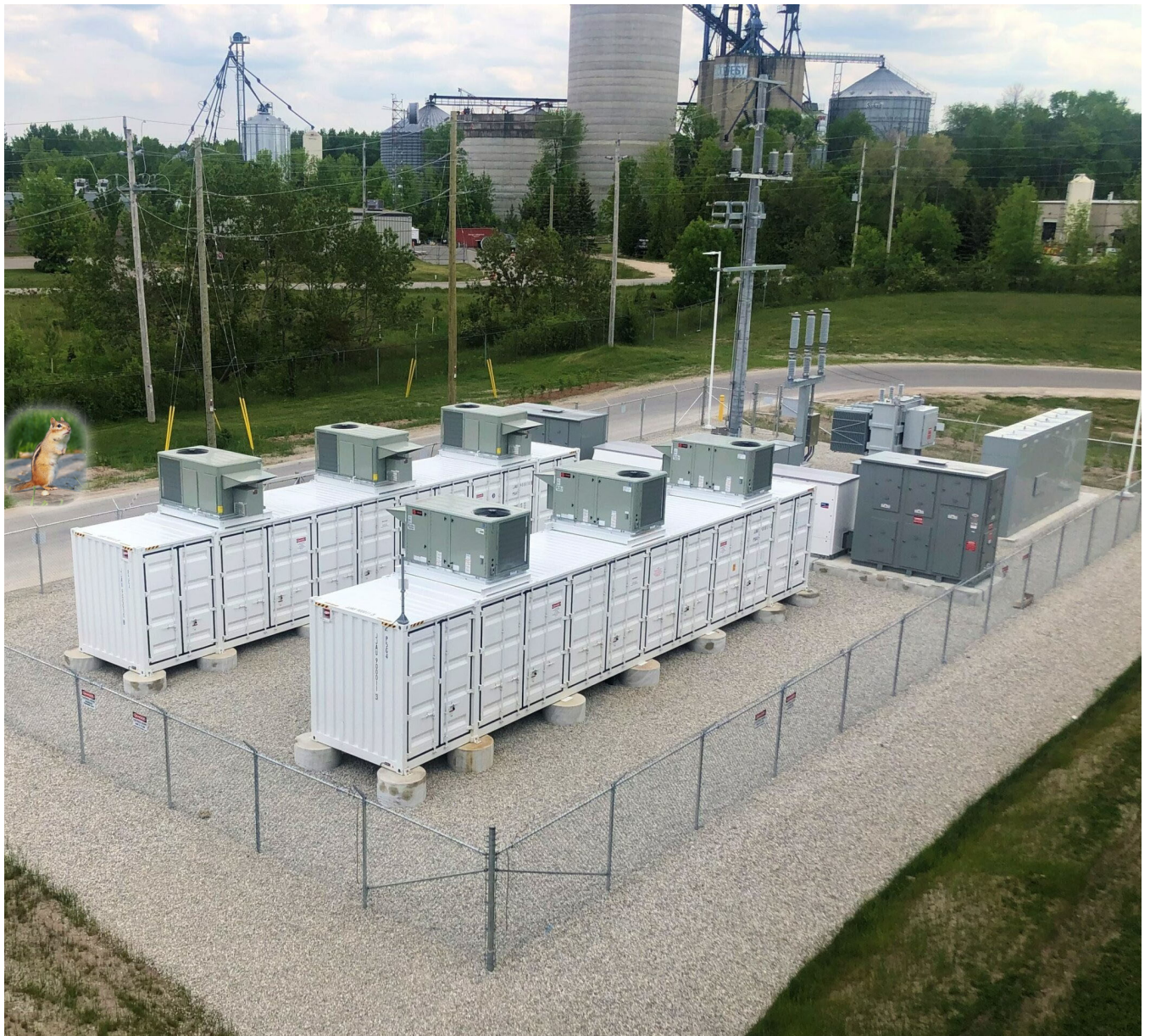
Example of a battery storage system
